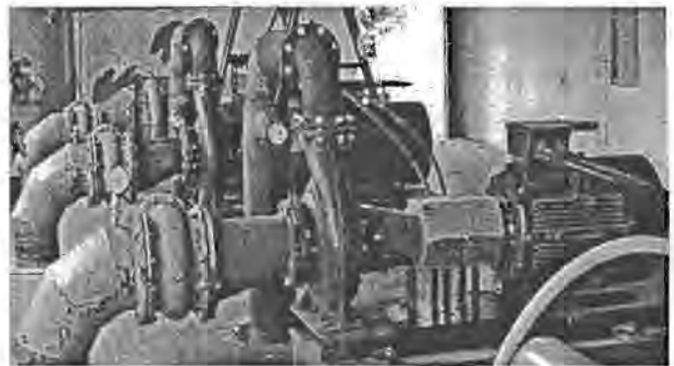
Figure 2. PS "Berilovac" after installation of another NK 150/400/380 pump (present state)
